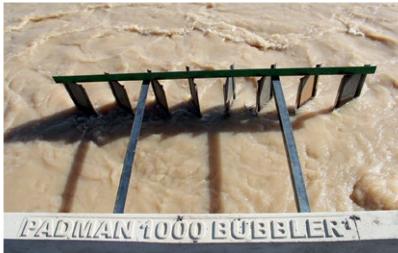
Figure 1: Padman Bay Outlet fitted with dispersion vanes.
