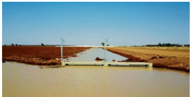
Figure 1: Head ditch structure – Padman Stops 2 x 1.5m.
